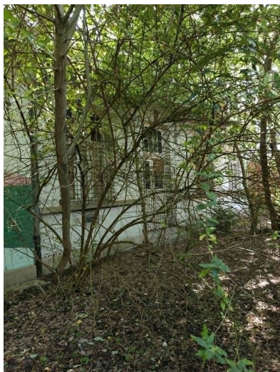
Cheminement quasi inaccessible
